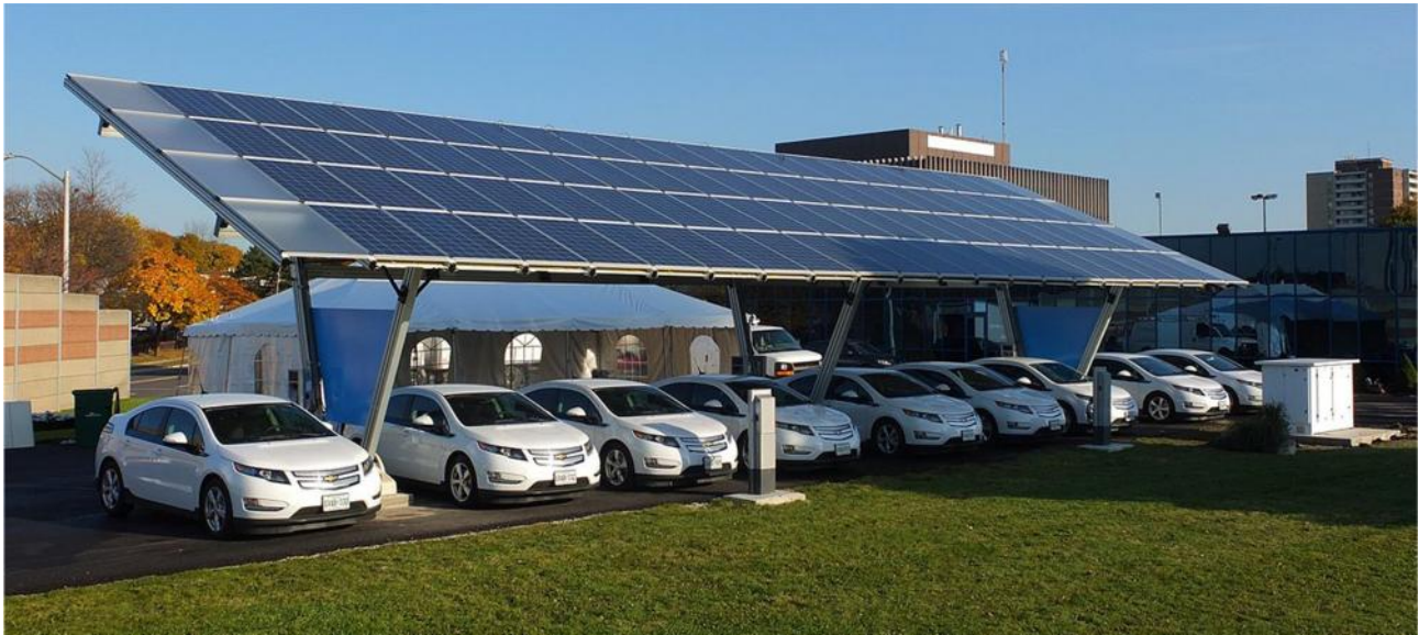
Green Mobility Station 20 kWp PV plants
